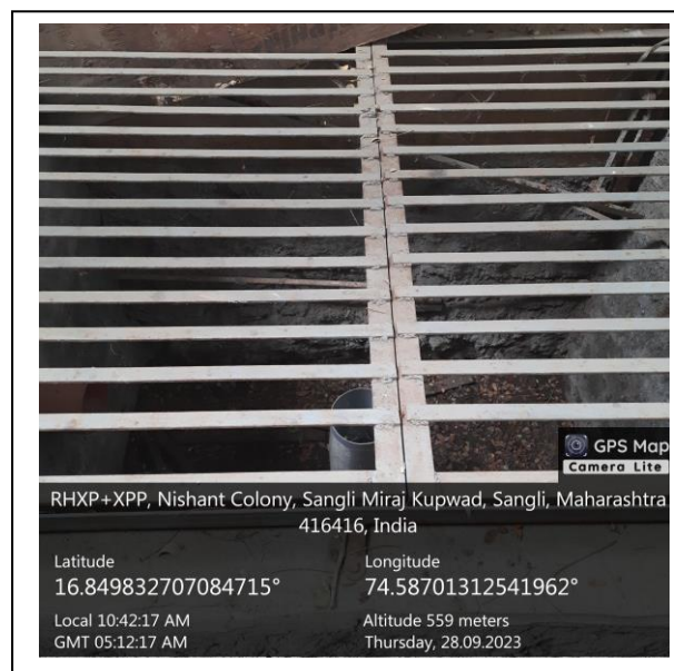
Rainwater Collection Pit
