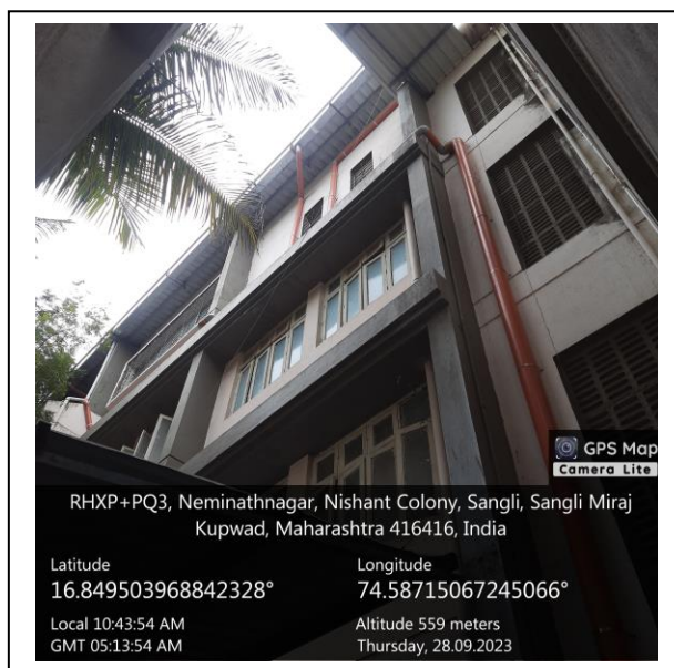
Rainwater Harvesting System
