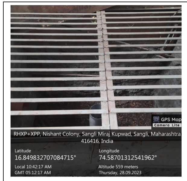
Rainwater Collection Pit
