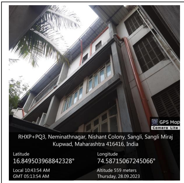
Rainwater Harvesting System
