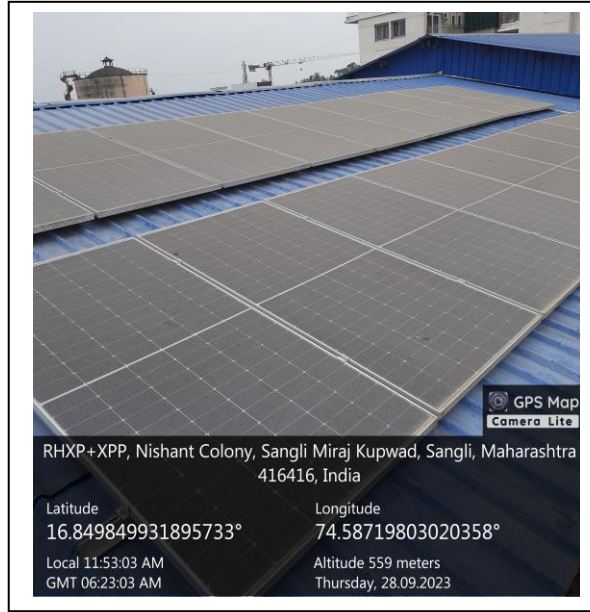
10 kW solar power plant
